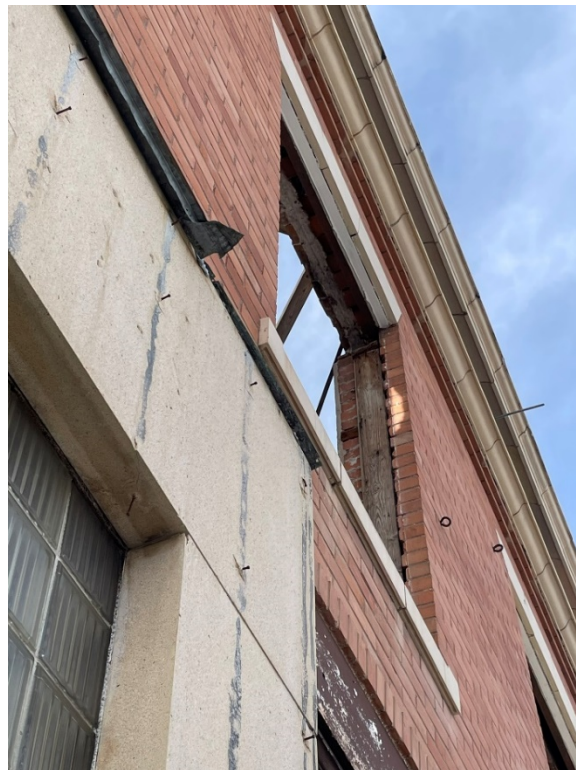
Photo 6 – Brick Support at Header Missing
