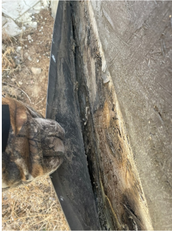
Photo 7 – Deteriorated Sheathing at Base of South Stabilization Wall
