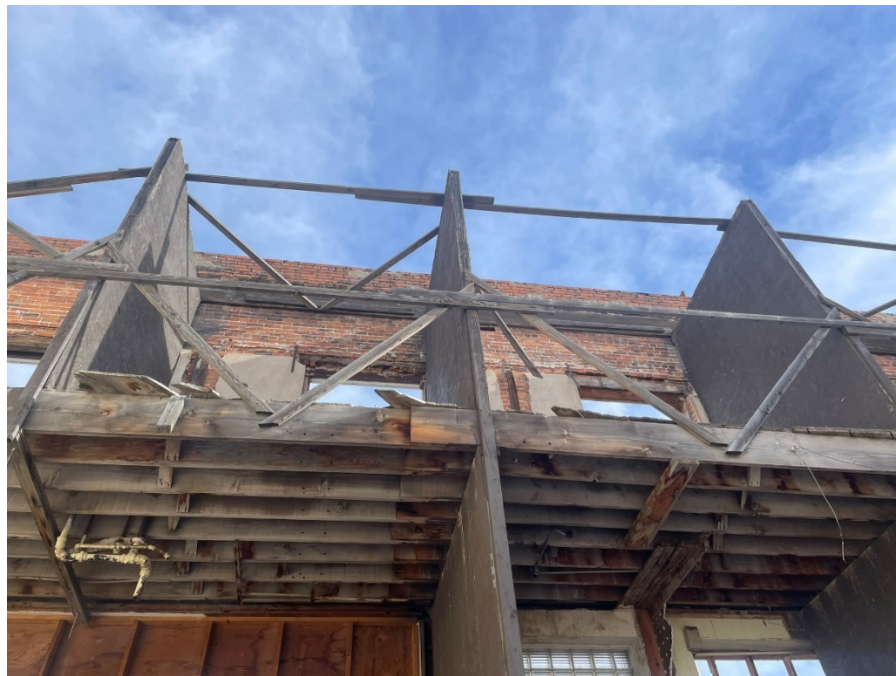
Photo 4 – Middle Portion of Stabilization System, Missing Cross Bracing, and Deteriorating Platform
