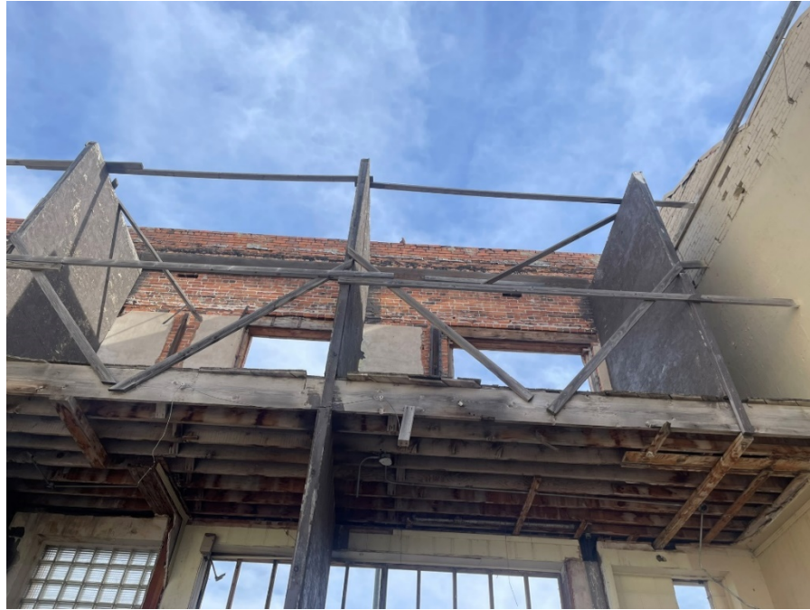
Photo 5 – South Portion of Stabilization System, Missing Cross Bracing, and Deteriorating Platform
