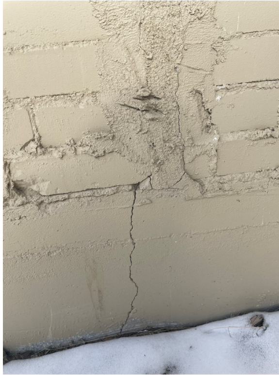
Photo 3 – Crack at Base of North Wall
